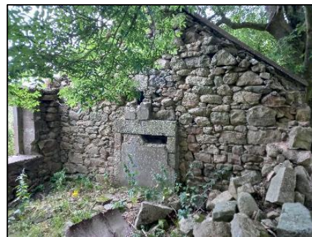
Photograph 6: Gaps between ruined building's stonework where masonry has deteriorated, between masonry and remnant roofline and gaps between ruined building's chimney flue and stonework
