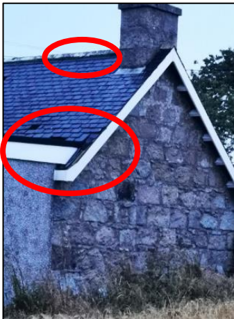
Photograph 3: Gaps under cottage roof slate and apex tile
