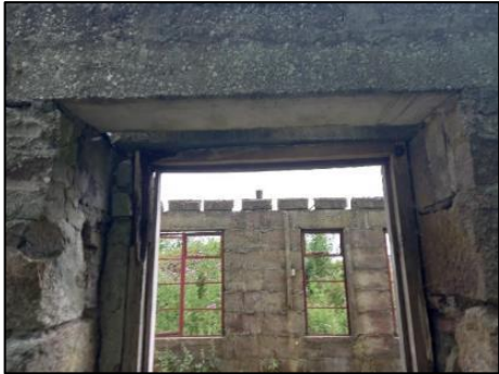
Photograph 7: Gaps in ruined building's wooden frame and stone lintel
